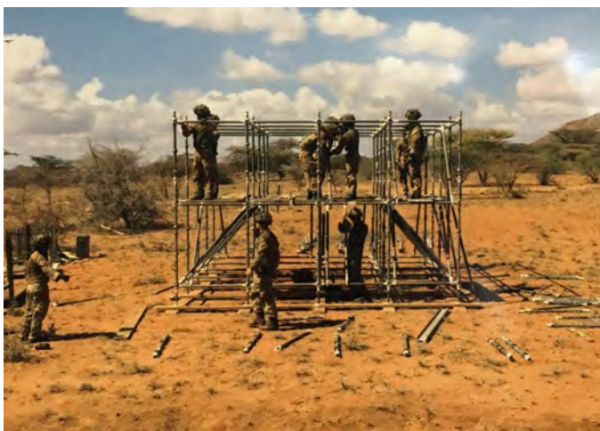
A cuplock tower being erected as a part of a BG Water Point
