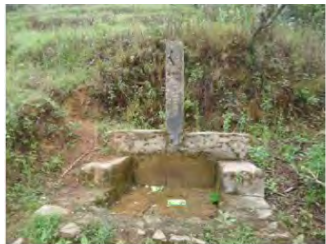
Condition off existing tap stand
