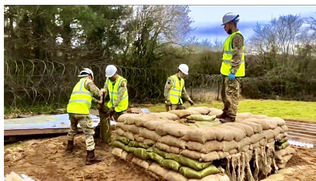
GPMG SF upgrading by APNR Members
