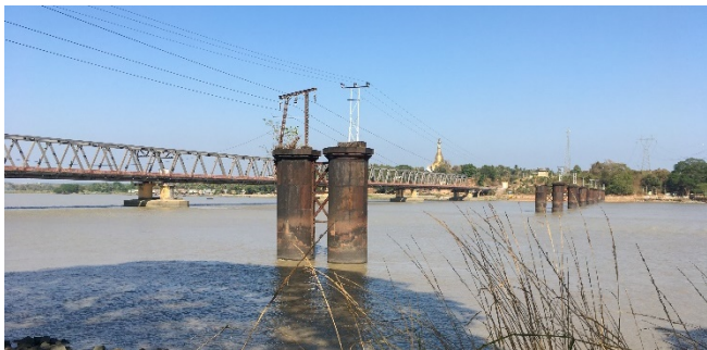
The demolished Sittang Bridge, looking south. The new replacement bridge is in the background
