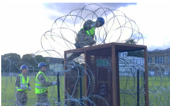
Close Sp Tp constructing Triple concertina wire fencing around a Network Equipment Room
