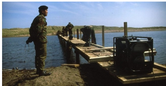
The bridge over the salt marsh at St Cyrus National Nature Reserve takes shape in 1985, courtesy of Gurkha engineers
